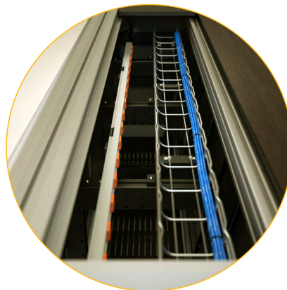
INTERNAL BASE POWER STRIP
